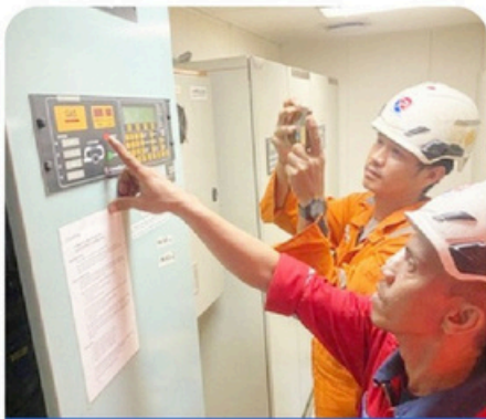
Fixed gas system calibration
