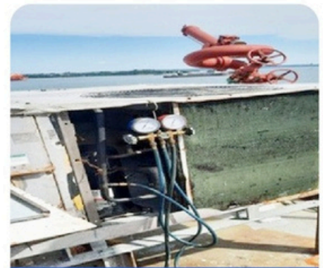
Inspection AHU system
