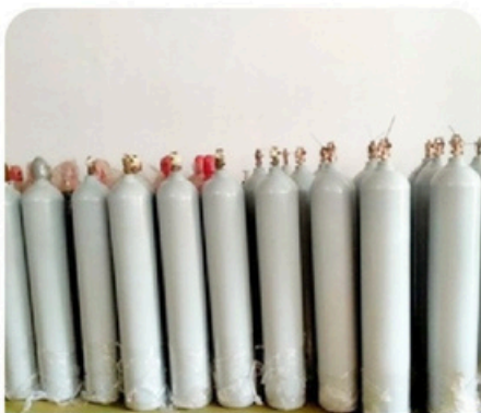
CO2 system before service
