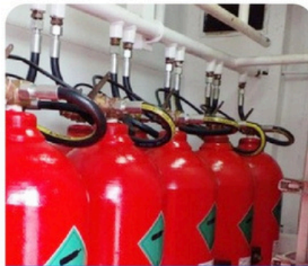
CO2 system after service
