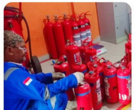
Fire extinguishers service
