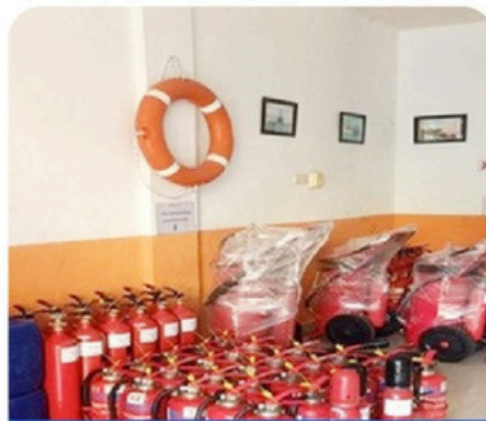
Fire Extinguishers after service
